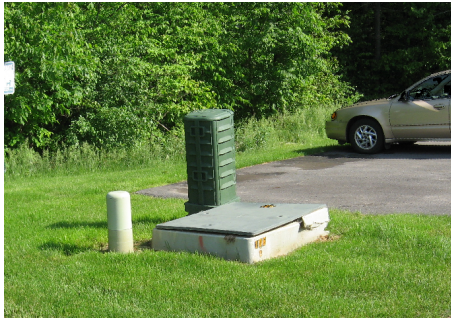
Figure 5.4: An electric box in a grassy field.
